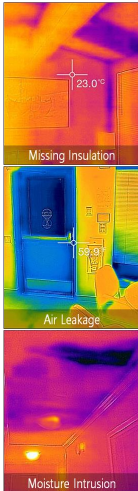
Figure 1: Common energy efficiency issues visible to a thermal camera.
